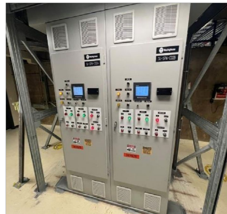
CE version of the MG control power cabinets installed
